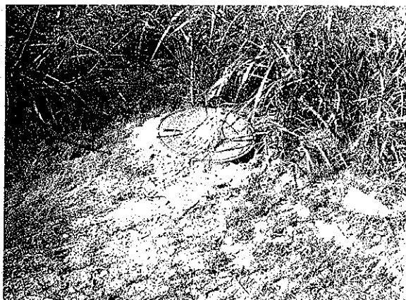
This area contains deteriorating infrastructure.
