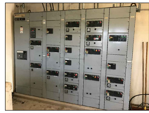
EXISTING MCC-1A PHOTO
